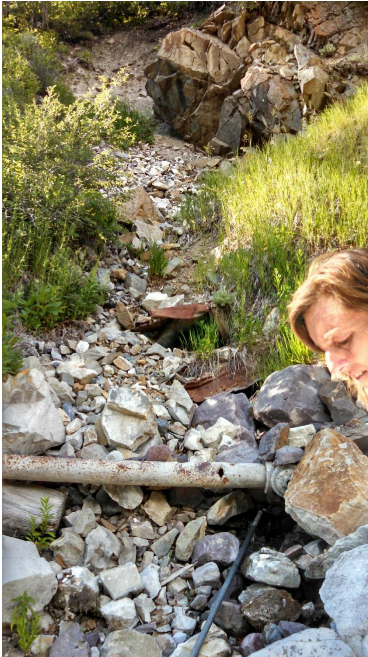
Figure 13 This pipe allows the James Drain tunnel to continue draining its water and is visible from the highway.
